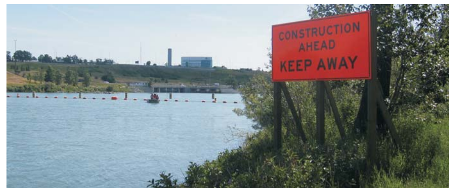
Looking down the Bow River at the safety booms upstream of the weir
